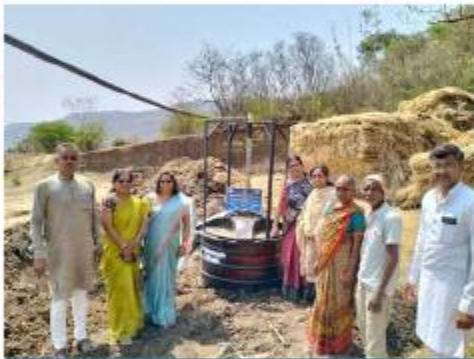
IWC NIGDI PRIDE INSTALLED 6 BIO GAS PLANT IN VILLAGE WORTH RS 1,40,000/-
